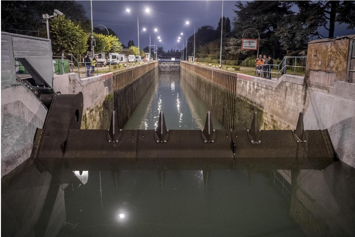
Figure 4 : Vanne de Saint Maur (source : CD94, copyright Michael Lumbroso)
